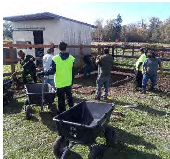
Digging and leveling out the ground to build concrete forms for the woodshed
