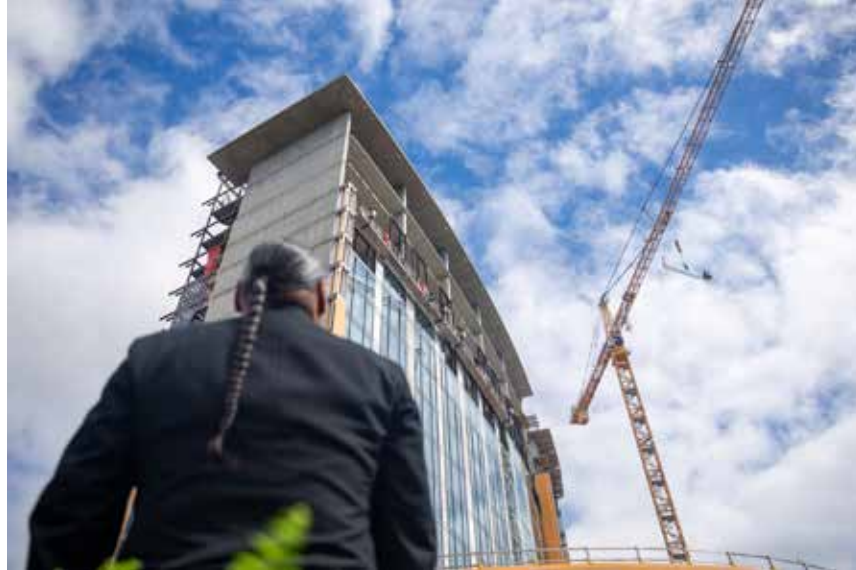
Muckleshoot Casino COO Tyrone Simmons watches as the final beam for Muckleshoot Casino's resort tower is placed atop the 18-story structure on August 26, 2022.
