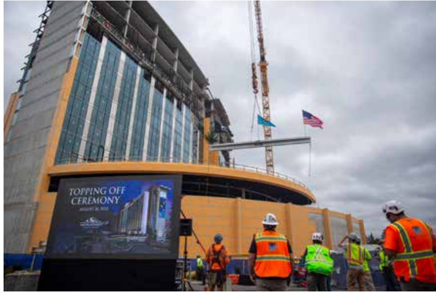
Construction workers watch as the final beam for Muckleshoot Casino's resort tower journeys to the top of the 18-story structure on August 26, 2022
