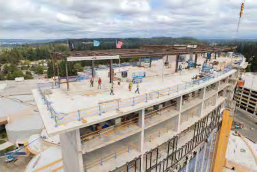
The final beam for Muckleshoot Casino's resort tower is placed atop the 18-story structure on August 26, 2022.
