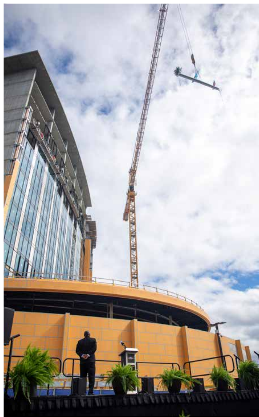
Muckleshoot Casino COO Tyrone Simmons witnesses the topping off of Muckleshoot Casino’s resort tower on August 26, 2022
